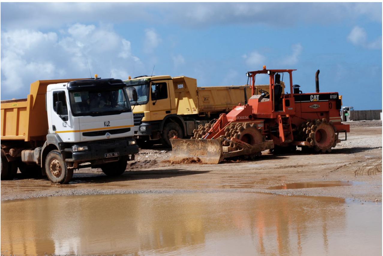
4. Construction of the platform for the mineral separation plant at the Mandena mine site.
